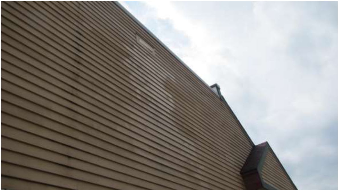
Wall wet from rain draining from scupper
