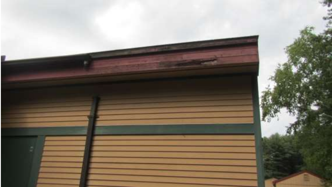
Water-damaged roof eaves
