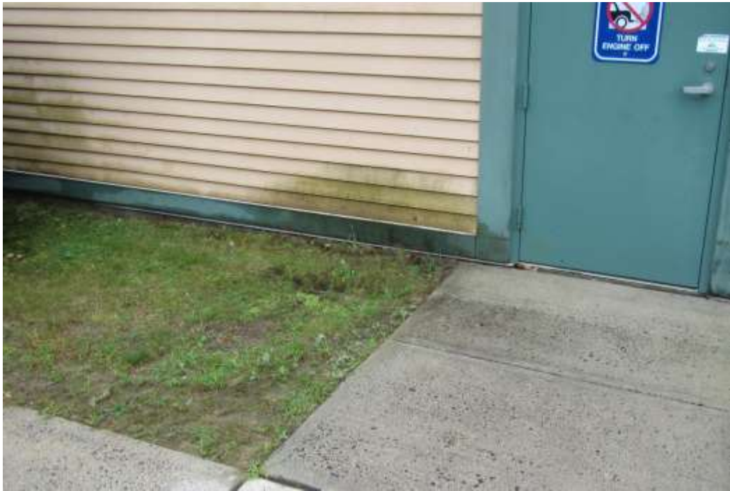
Moss on exterior walls
